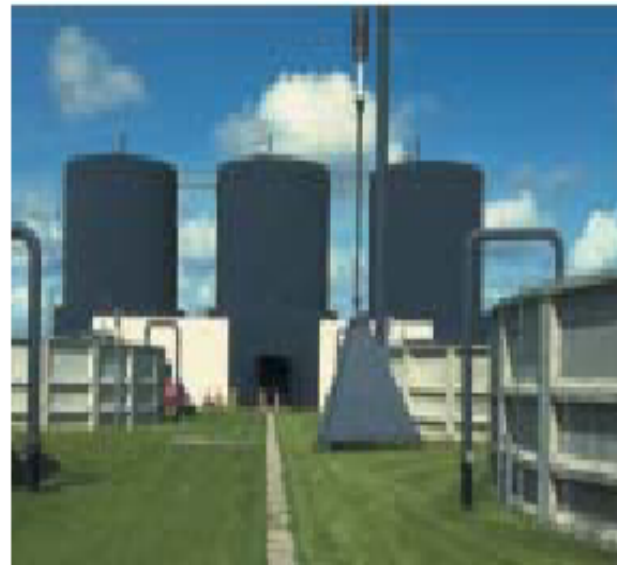
Large Scale Centralised Co-digestion Plant Lemvik, Denmark (Picture courtesy of Teodorita Al Seadi, Denmark)
