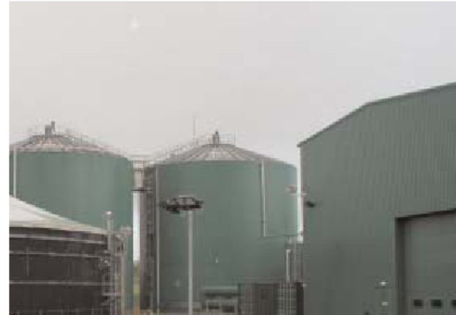
Large scale co-digestion plant, Holsworthy, UK (Picture courtesy of Rudolf Braun, Austria)
